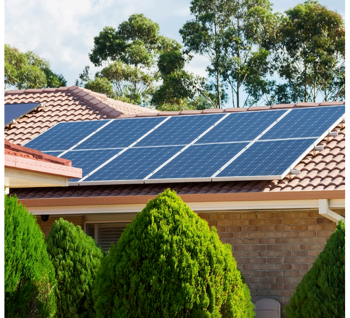
Make the most of your rooftop solar investment: Do your research and follow best practices.
